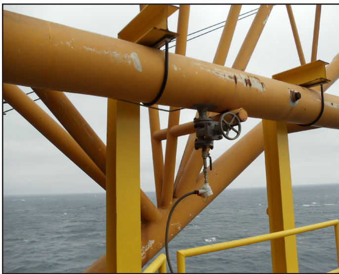
Fox Model FT3 in a remote configuration used to measure flare gas at an offshore drilling rig.
