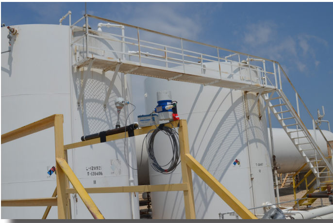
A portable Fox Model FT3 kit used at oil and condensate storage tanks for emissions requirements.
